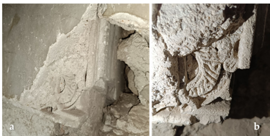
Figure 7. Fragments of plasterworks in the qibla wall. Photograph by Sergio Ramírez González.
