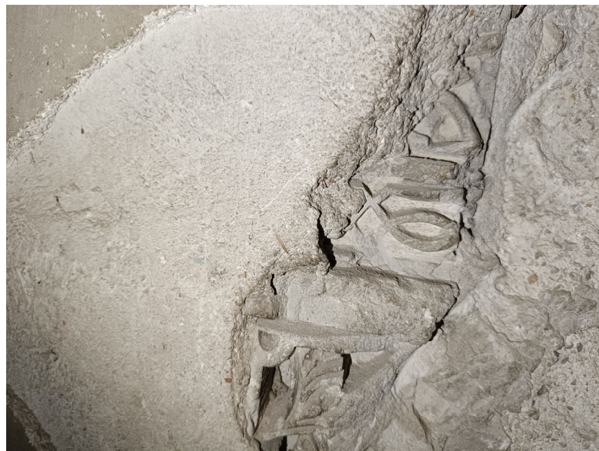
Figure 12. Fragments of plasterworks in the qibla wall. Photograph by Sergio Ramírez González.
