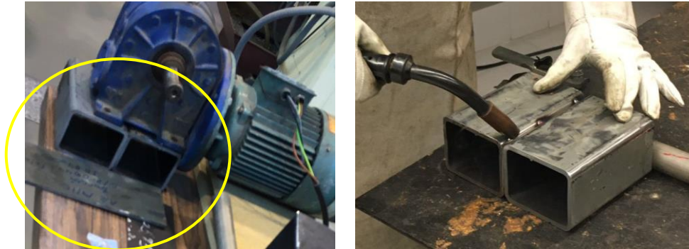
Fig. 2. Geared motor assembly for MAREA Plastic extruder with supporting structure (two welded quadrangular section profiles).
