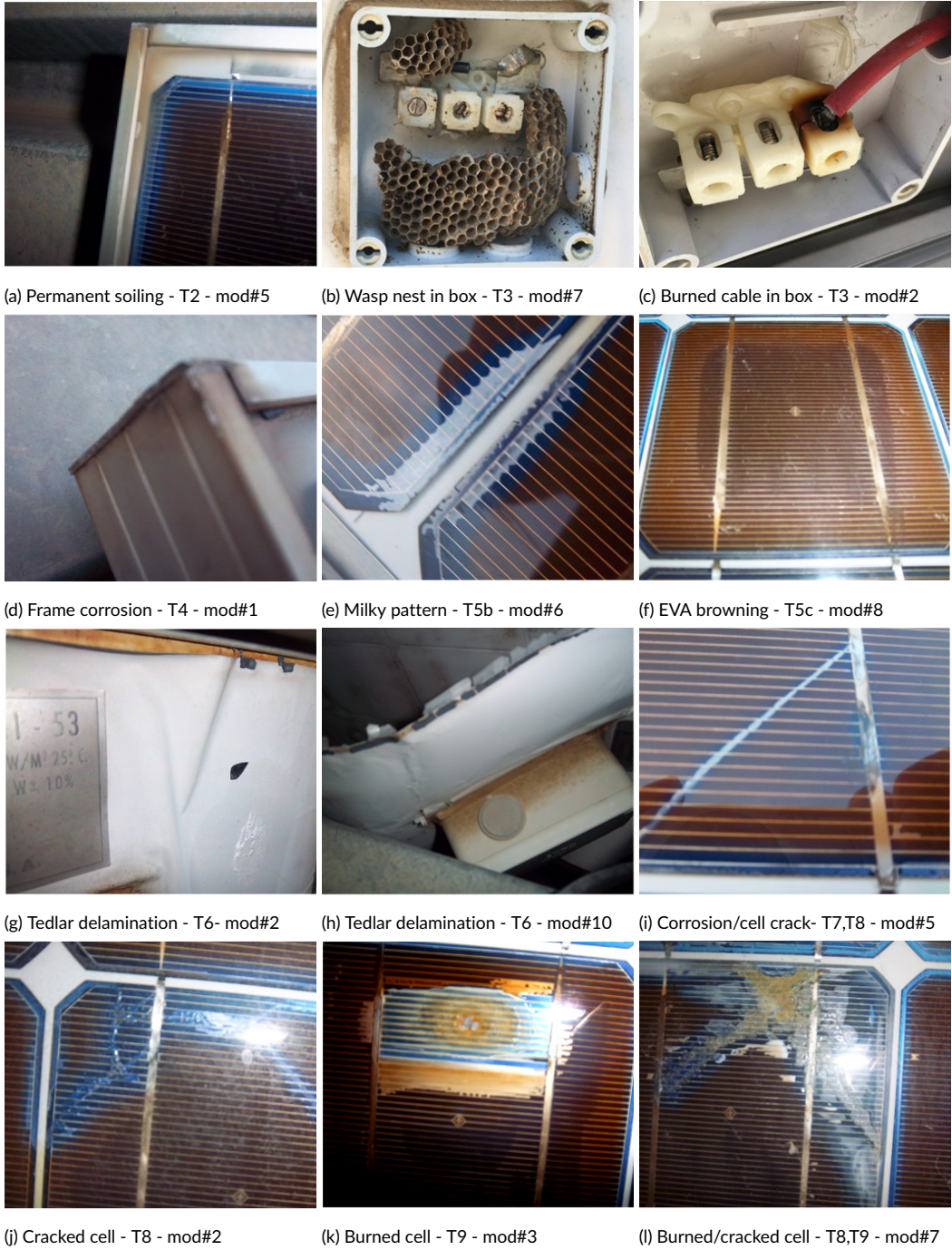
FIGURE 2 Result of the visual inspection of the modules under study.
