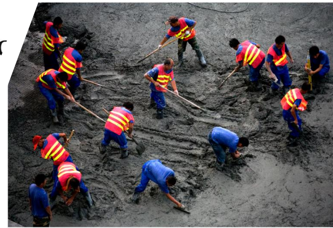
Workers cement a road, demand for cement for infrastructure is projected to grow significantly. REUTERS/Kevin Coombs Purchase Licensing Rights
