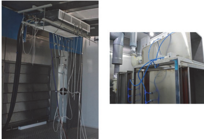
Figure 2. Chilled beam in the test chamber (left) and nozzle bank for air flow measurement (right)
