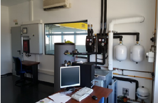
Fig. 1. Laboratory of Cogeneration.
